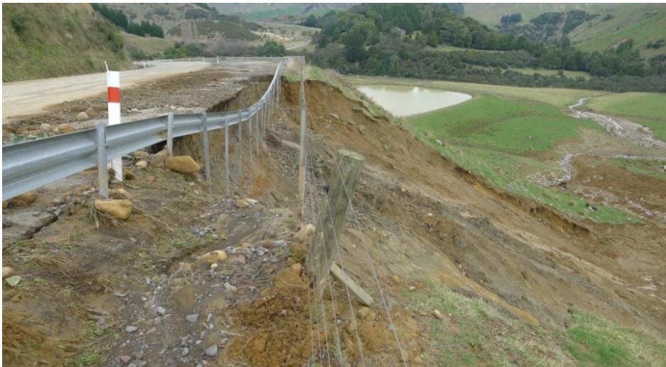
SH 4 at RP148 slip and guardrail storm damage
