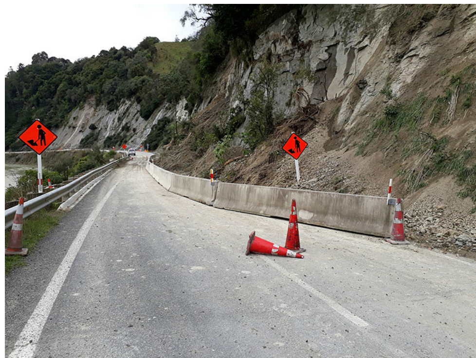
Slip north of Fields Track at the Hapokopoko Bluffs, dumped approximately 500m3 of material onto the road.
