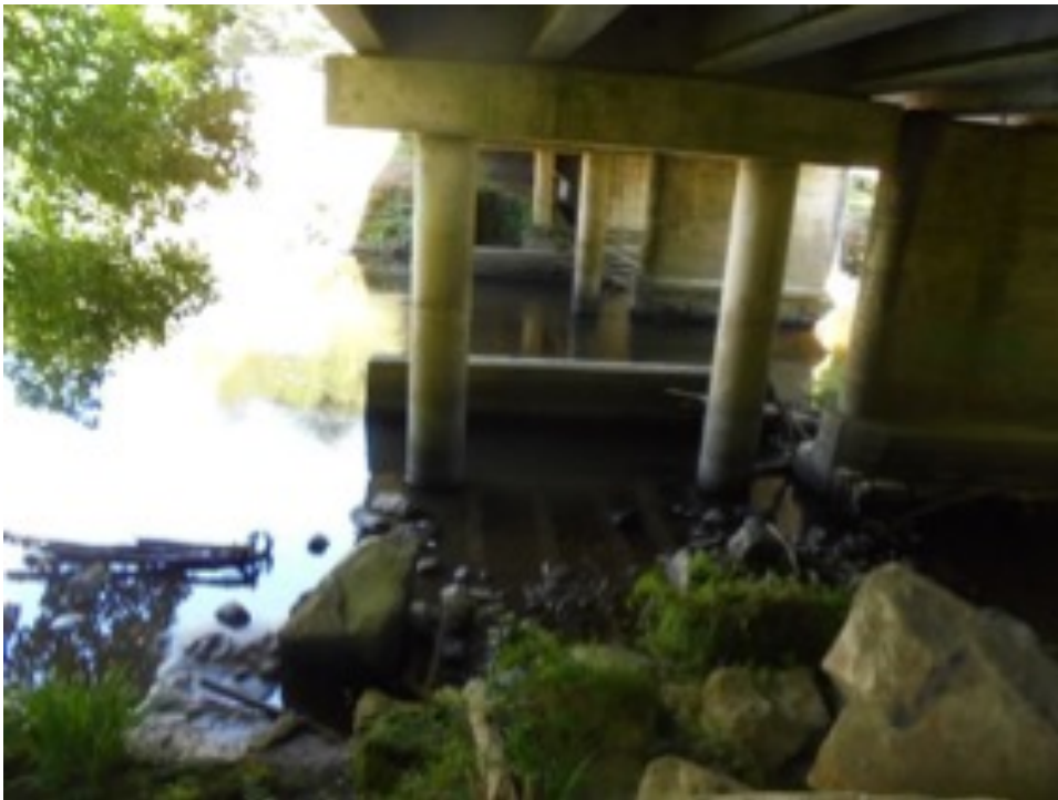
Ongarue River Bridge exposed abutments
