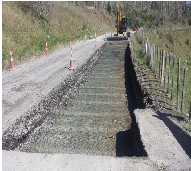
SH 4 at RP 158, rip and remake slow slip movement site
