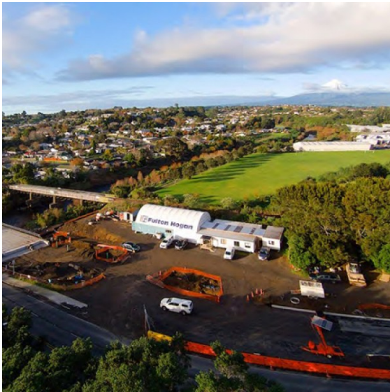
Improving capacity between Vickers Road to Hobson Street on State Highway 3, New Plymouth.
