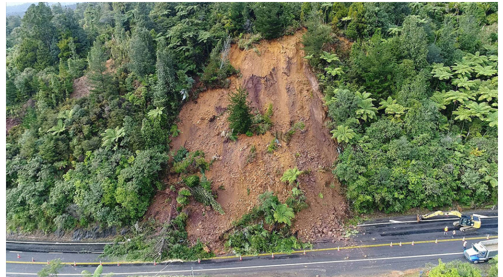
2.5 metres of rain fell on the hills of the Coromandel Peninsula causing slips on SH25
