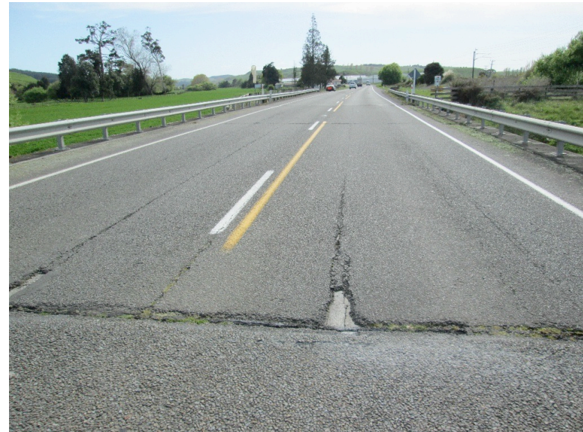
Failed longitudinal & transverse joints on SH1 Porewa Stream (Rata Station) Bridge
