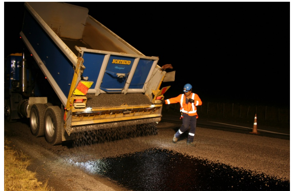
Maintenance work is scheduled at night to minimise travel interruptions to customers
