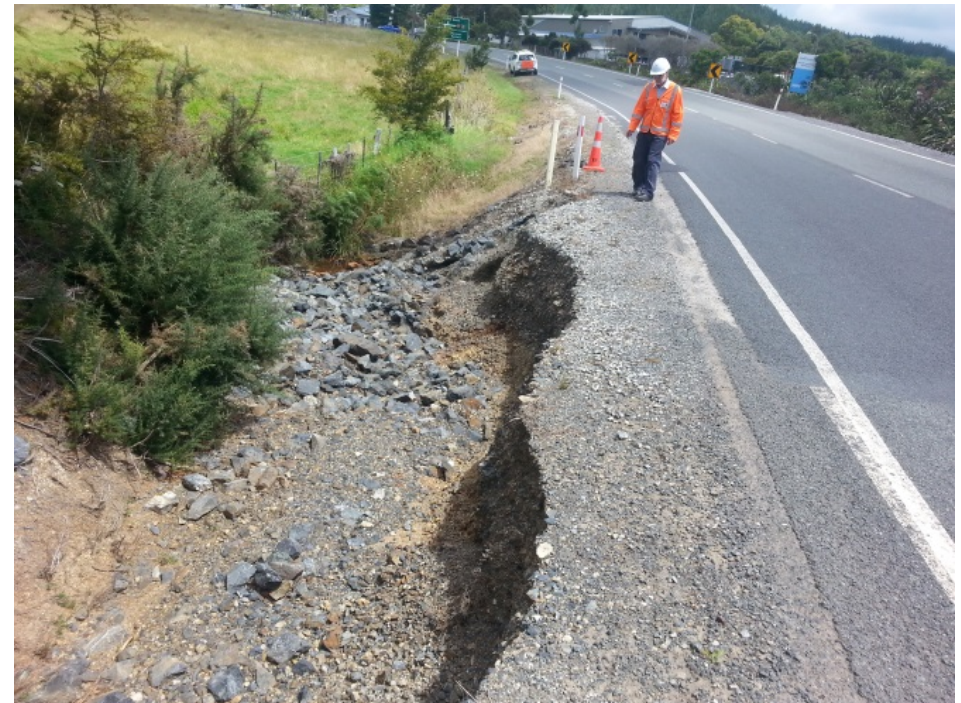
Under slips can quickly undermine the pavement
