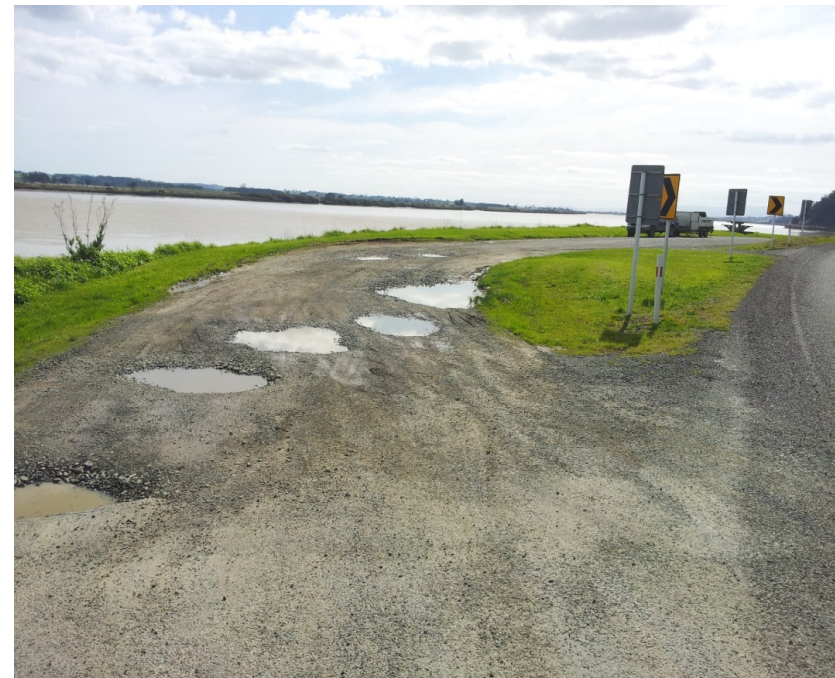
Tokatoka Bluff rest area maintenance needs
