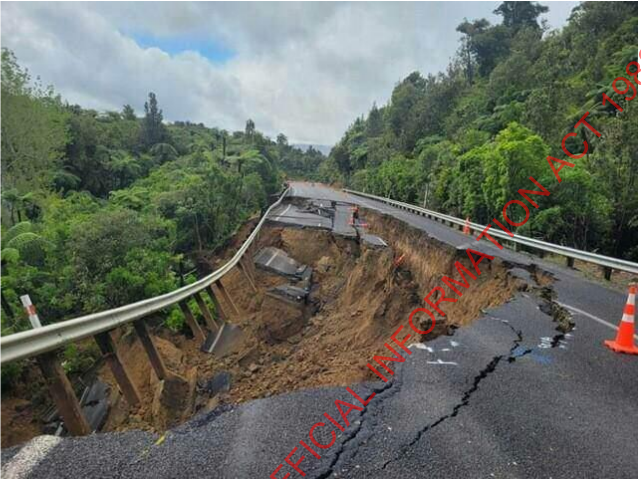
Figure 3.2 – First failure of the embankment on Saturday 28 January 2023.
