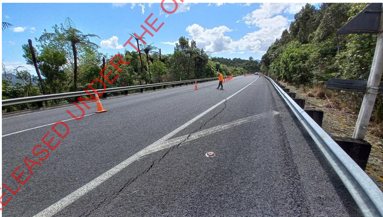
Figure 3.1 – Initial cracking of pavement observed on Monday 16 January 2023.
