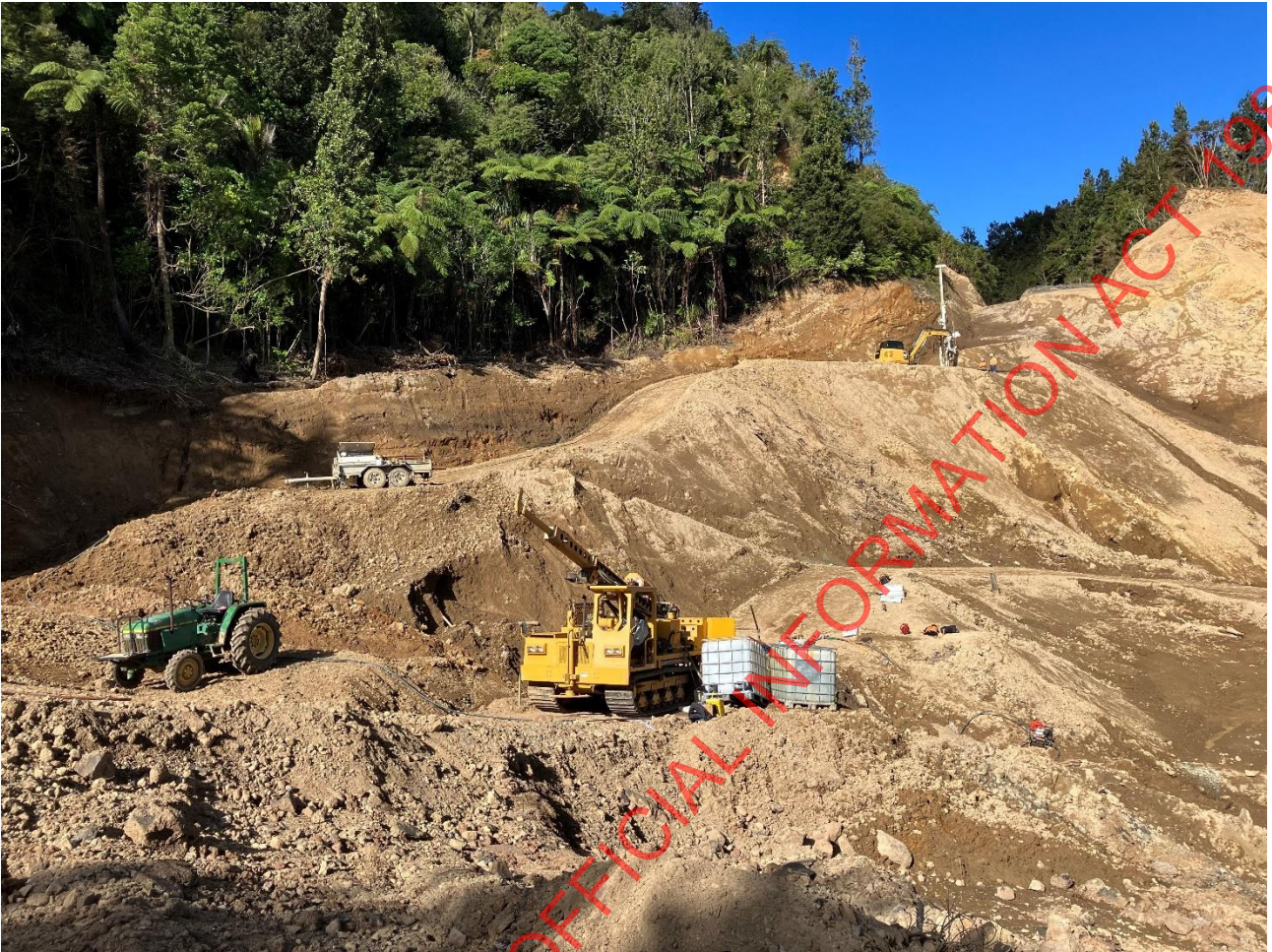
Figure 3.4 – Current condition of the slip scarp. Photo taken during geotechnical investigations 29 March 2023.
