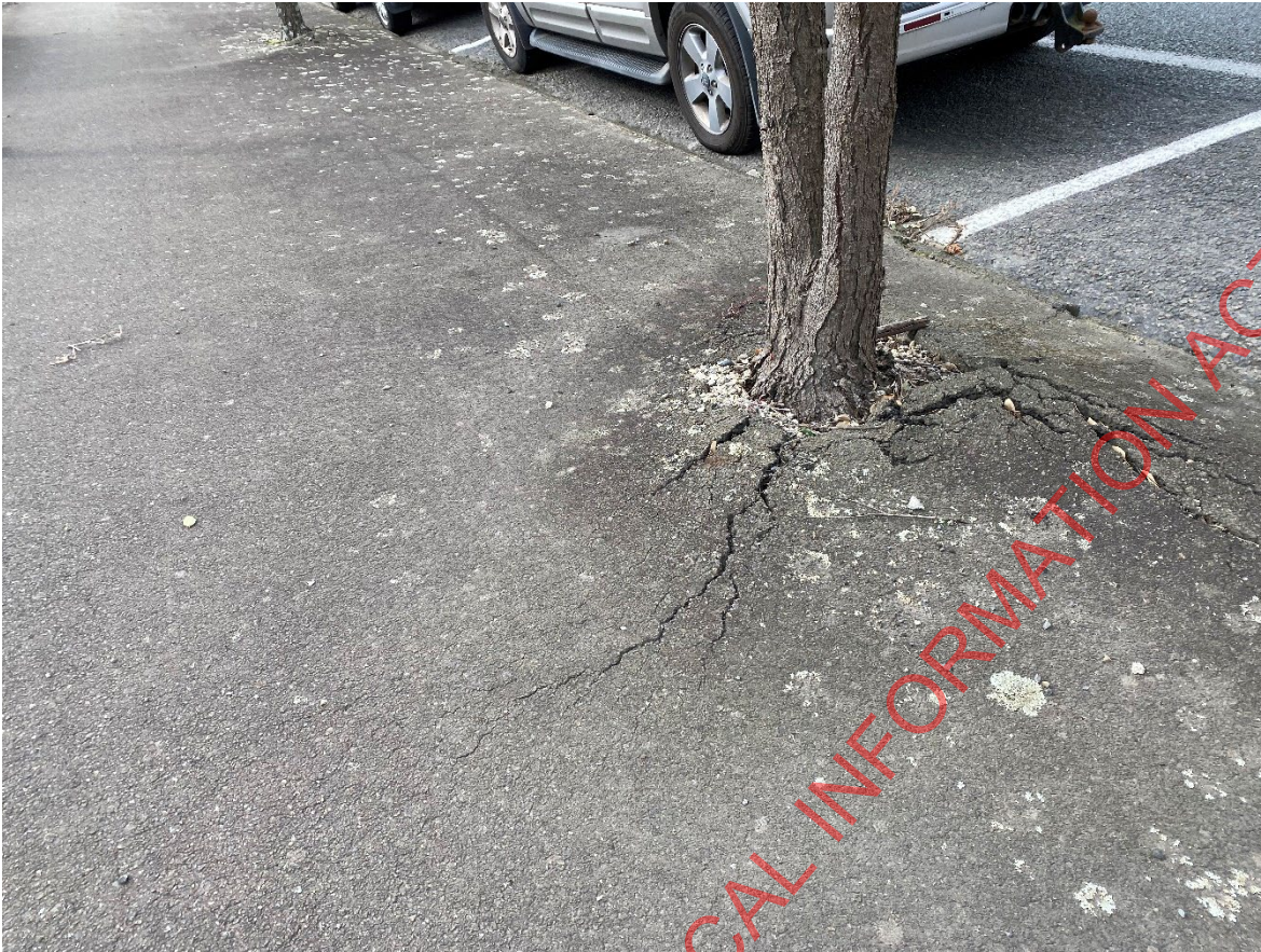
Figure 22: Existing uneven path adjacent to Hutt Road.
