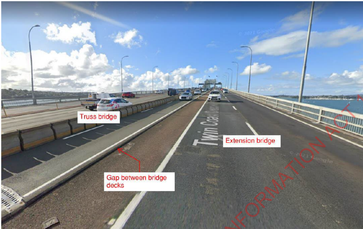
Figure 2: Gap between bridge decks
