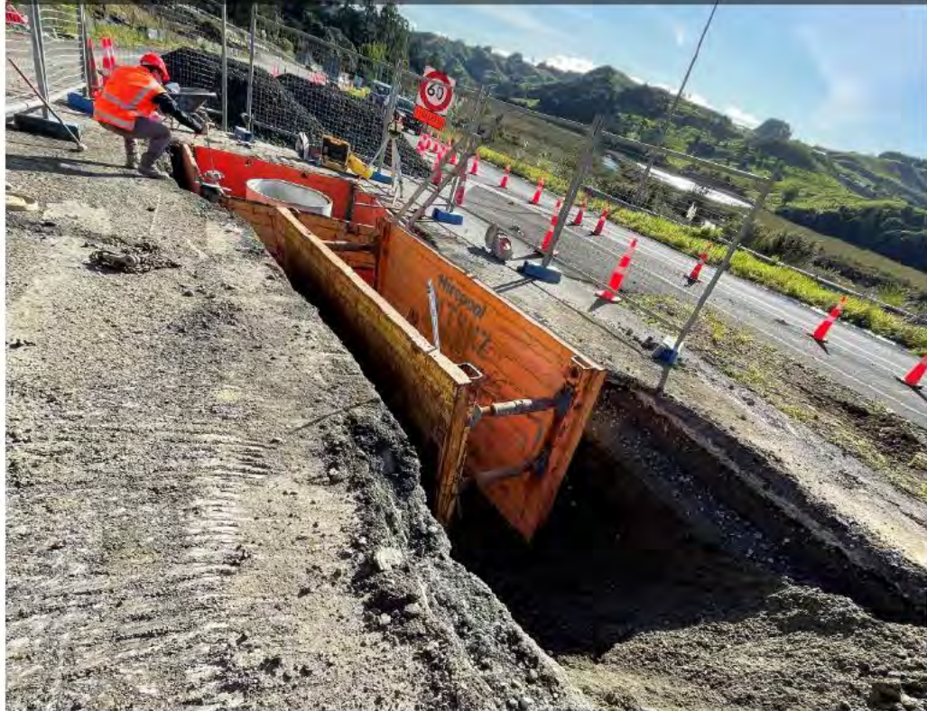
Southern tie-in: Manhole installation and existing stormwater pipe upgrade, ch.65000 (looking north)
