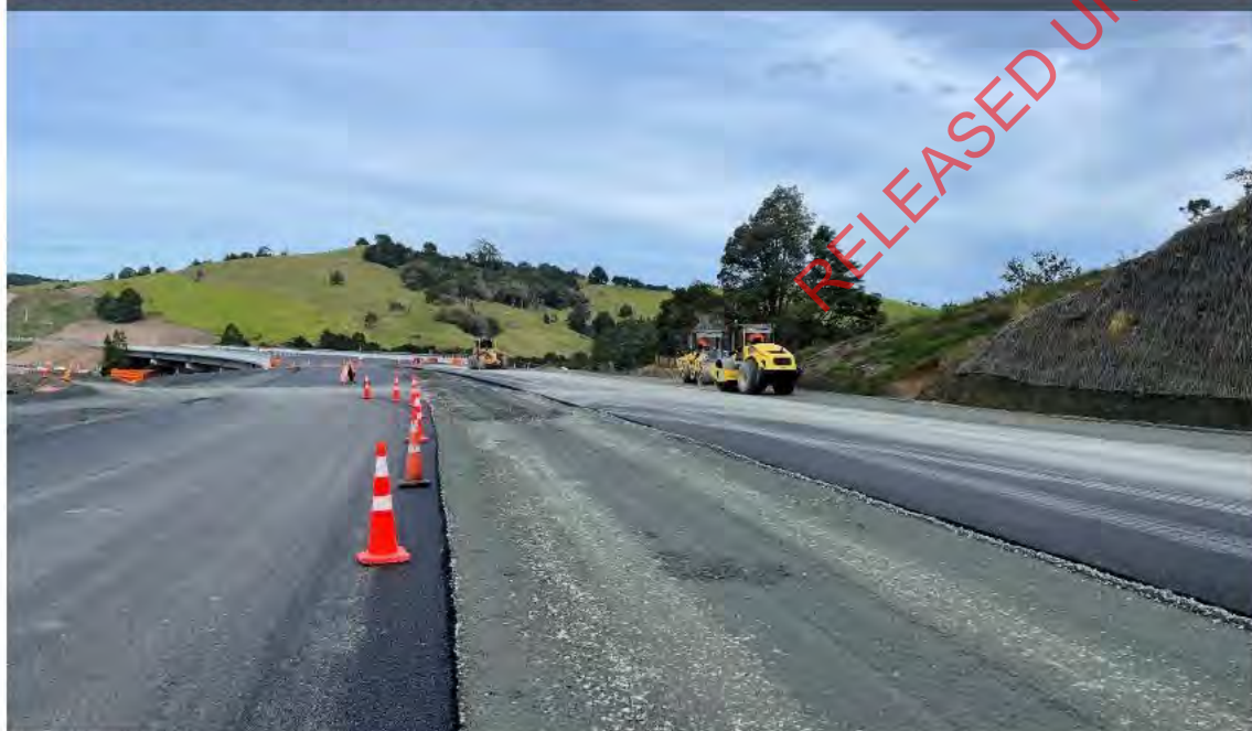
CS16d: AP40 stage 2 placed and compacted along median and shoulders, ch.62500 (looking south)
