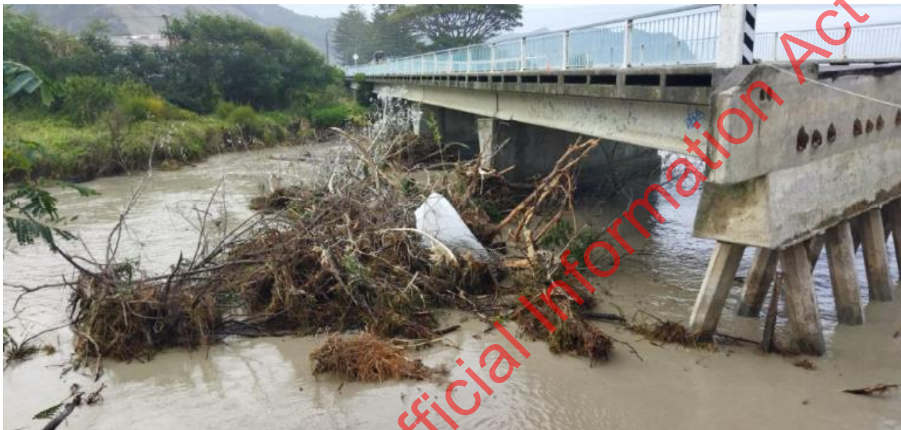
Figure 2-1 : Woody debris upstream of southern end span. (Failed abutment approach is at RHS)
