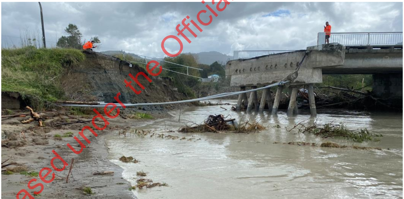
Figure 1-2: Looking upstream, showing washed out abutment and gap to the road
