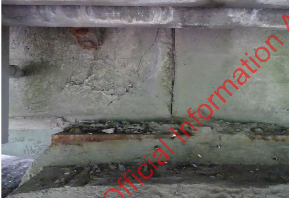
Figure 3 - Cracking at beams ends like due to thermal movement (lack of appropriate sliding surface) and exacerbated by water leakage
