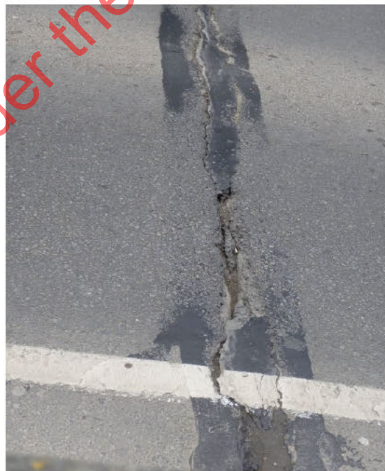
Figure 2 - Typical deterioration of deck joints, showing breakup and leakage.
