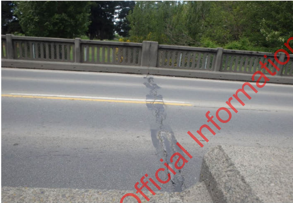
Figure 1 - Typical deterioration of deck joints
