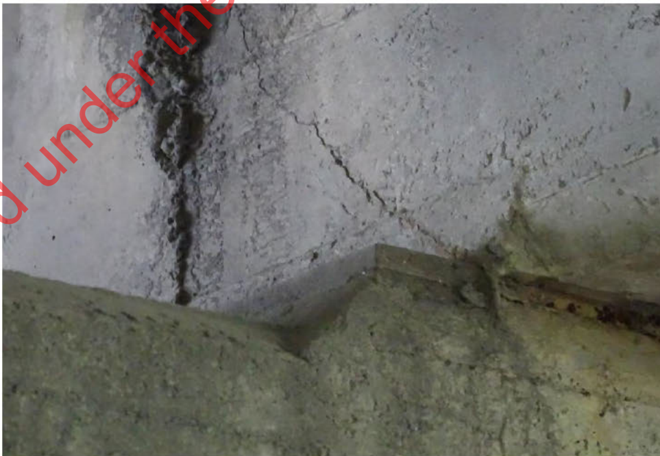
Figure 4 - Cracking at beams ends like due to thermal movement and exacerbated by water leakage. Could lead to spalling and seating
