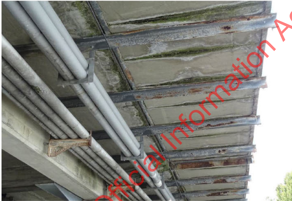
Figure 5 - Typical corrosion of footway joints. Will require recoating in a few years (at risk of section loss in a few areas).
