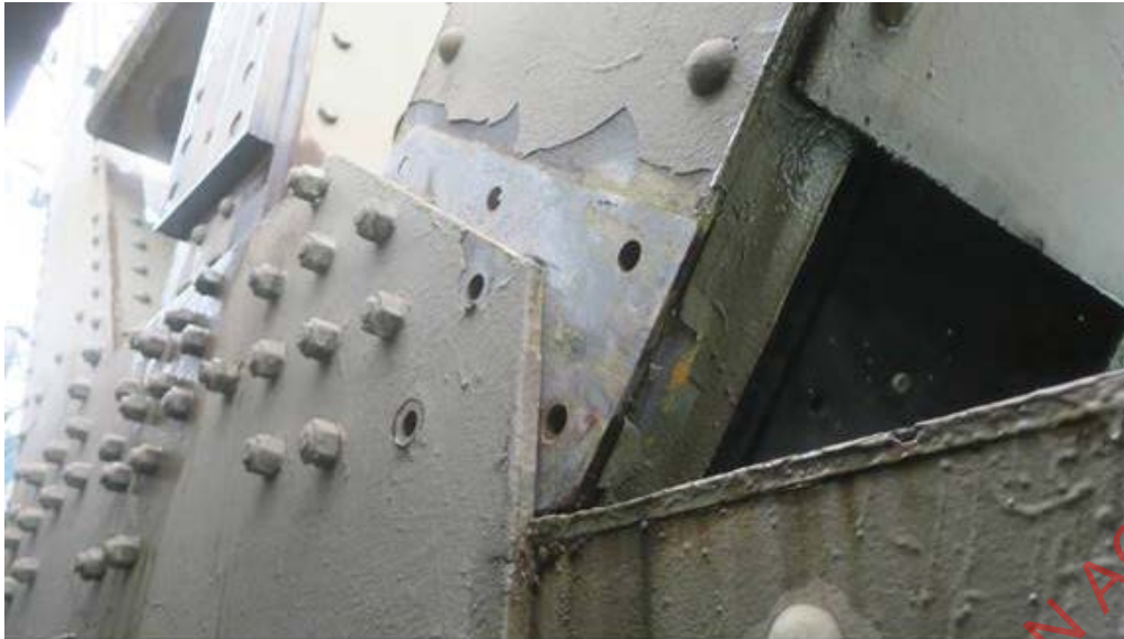
Caption: The bracket where the bridge truss has been sheared away, breaking the bolts holding it in place
